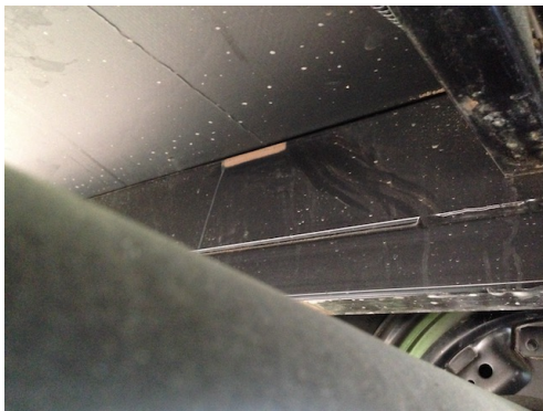
Rust high on the frame on the camp side in front of the axle.
