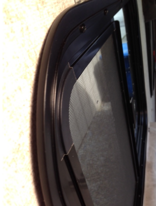
Photo 2 & 3: Gap on inside of kitchen window on the left side, not the side that is leaking.
