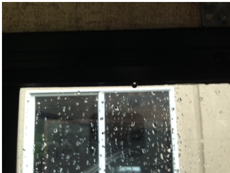
Photo 5: Top, right pane inside kitchen. A large drop can be seen on the inside and a smaller drop on the inside, just to its right. Small drops are on outside of window.
