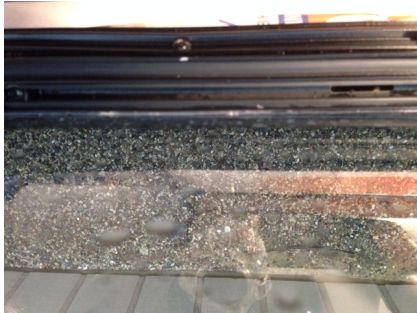
Photo 8: Goopy stuff can be seen on bottom of window pane, and I did not put it there. The goopy stuff looks like light or white scratches, but it is some kind of caulk.
