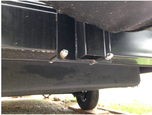
Rust on the lower, outside area of the spare tire bracket.
