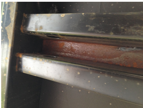
The photo shows rust on the camp side between, and on, cross-members.
